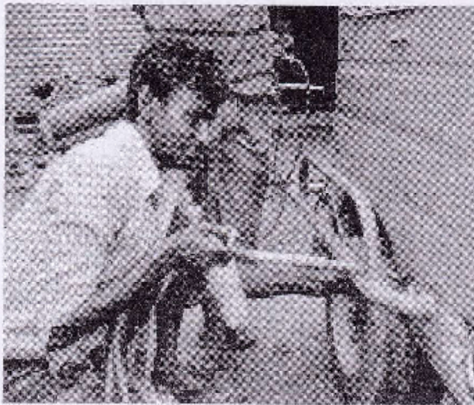
Fig.1: Worker is doing gas welding without safety
